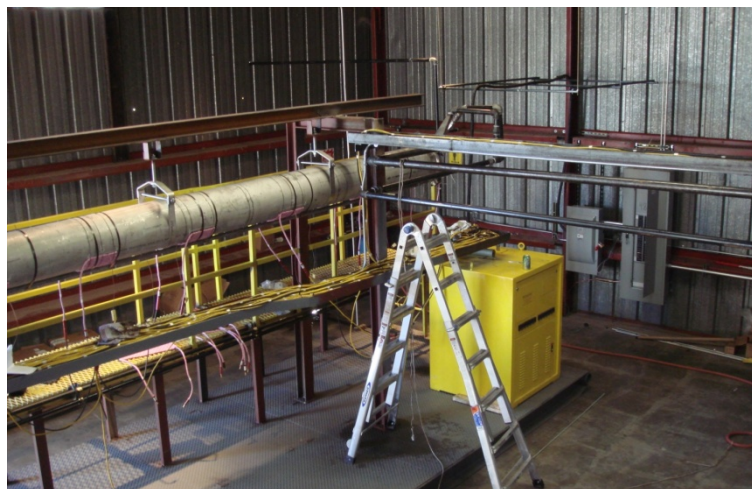
Figure 7. Overall view of the main upgrader reactor during assembly. Heavy crude enters the reactor on the right and proceeds toward the discharge on the left.
